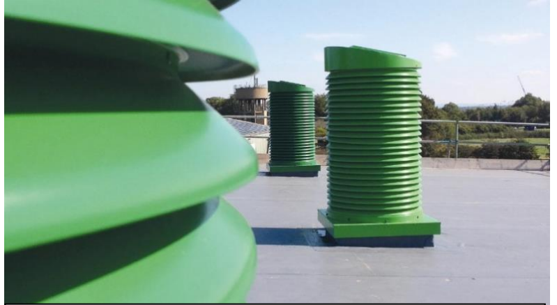
Figure 5- turrets on the roof of Askham Bryan Animal Management centre (Air distribution specialists, 2016)
